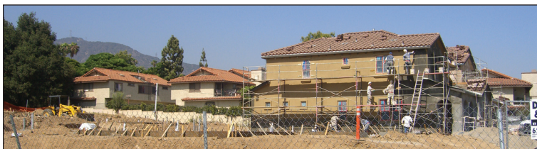
MODEL HOMES on the Bowden development project across from City Hall are set to be completed within the next several weeks. A total of 17 homes are being built on the site.
